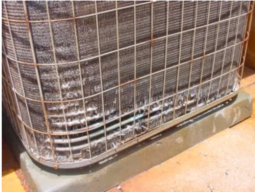
Figure 7. Deteriorated Area of Adsil Coated Condenser.
