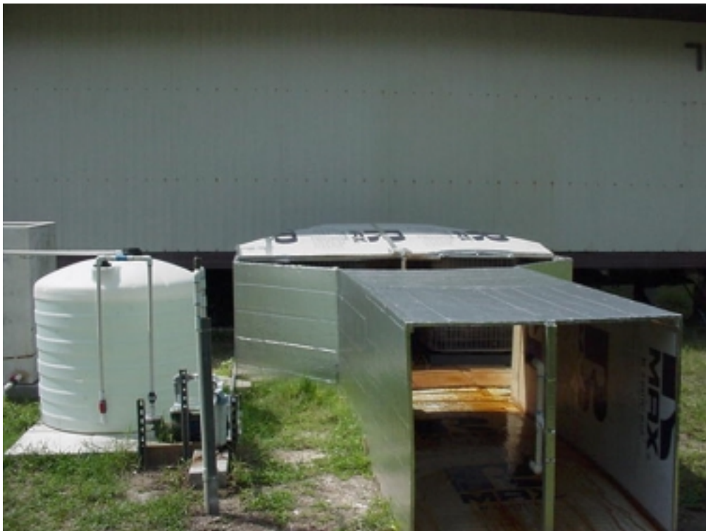
Figure 4. View Down Condenser Ducting and Salt Solution Holding Tank.
