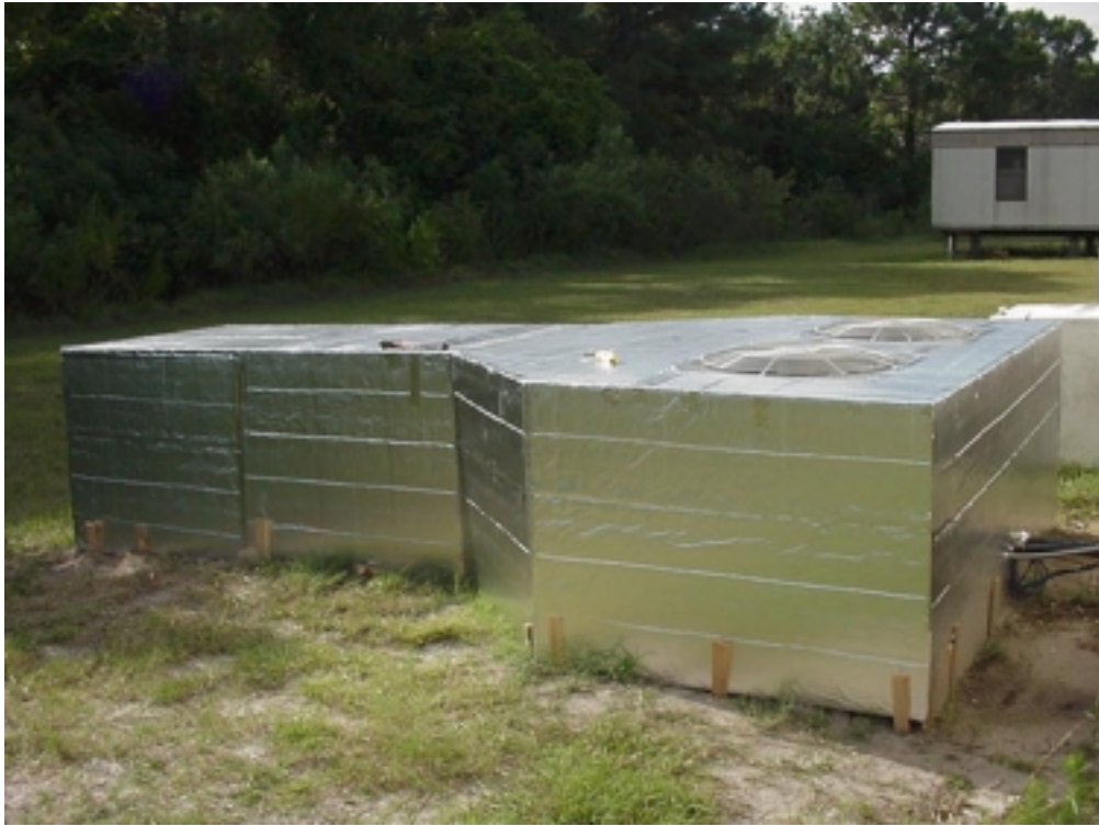
Figure 3. Ducting Constructed around Side by Side Condenser Units.
