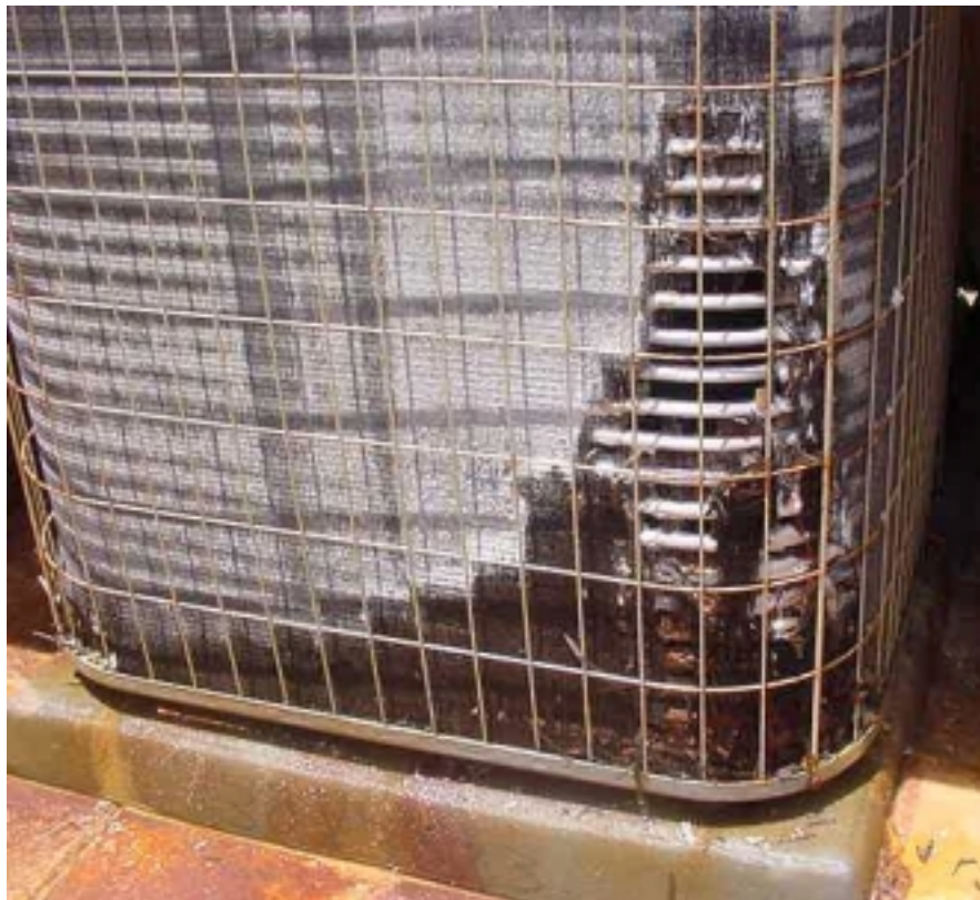
Figure 8. Portion of Deteriorated Area of Control Condenser.
