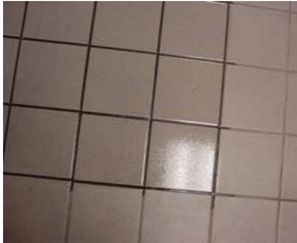
Glazed Tile Bathroom Winn Dixie Distribution Center
